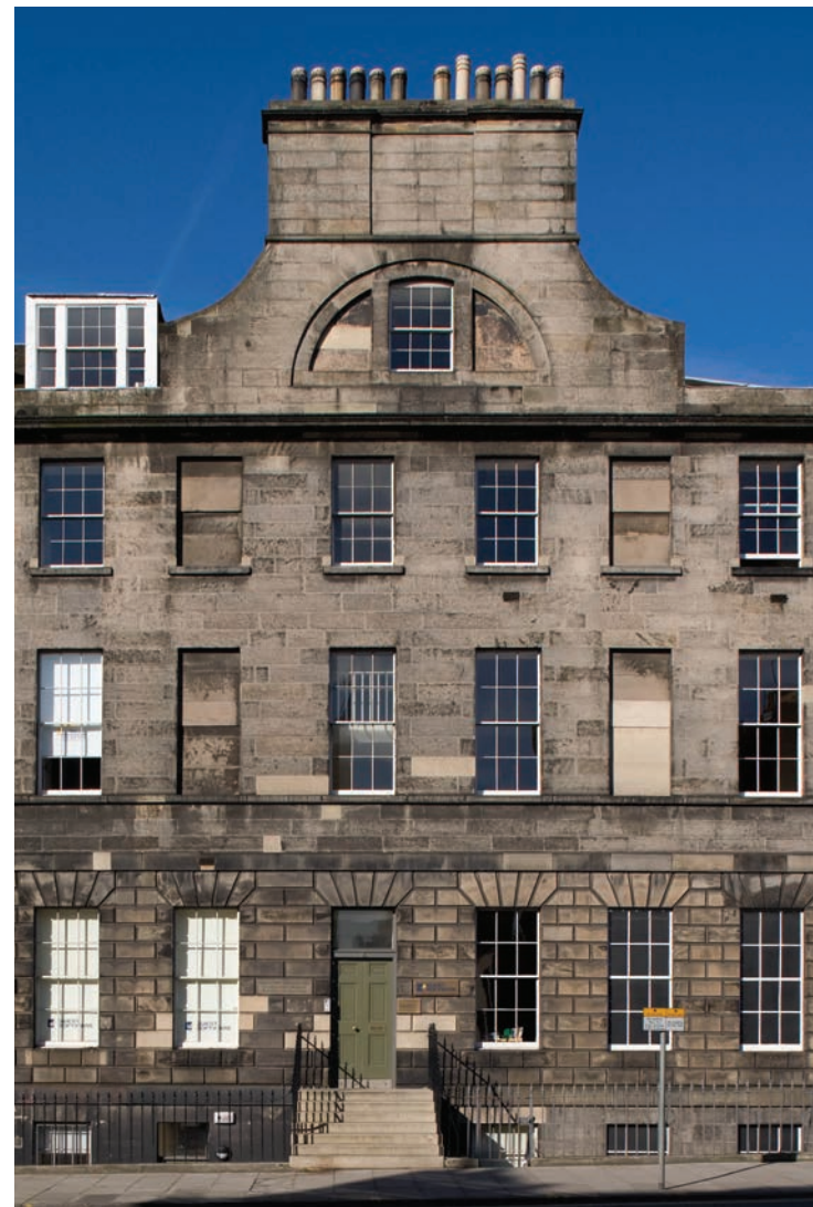
South Charlotte Street, Edinburgh. The blind openings are detailed with cills and a meeting rail to maintain the symmetry of the architectural elevation. There are chimney flues behind them within the walling.
